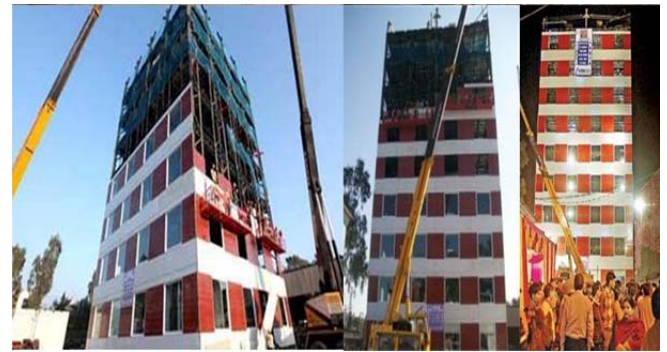
Fig. 1: The complete construction process photographs of the "10-floor 'Istacon' sky scraper at Mohali within just 48 hours". (Sources; download the picture form http://www.21stcentech.com
