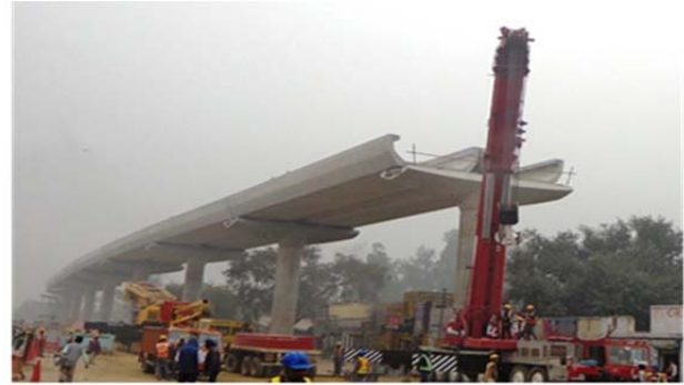
Fig 4. Under construction U-shaped full span segmental bridge. (Sources; visit the site and click the photograph)
