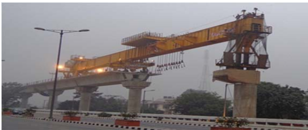
Fig3. Construction process of segmental bridge.(Sources; visit the site and click the photograph)
