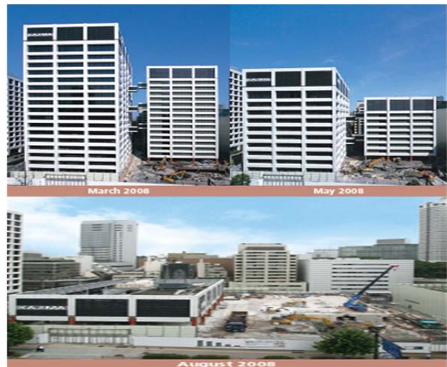
Fig. 9 Kajima DARUMA technique of demolition of tall buildings (Sources; the pictures are pick from the reference [8])
